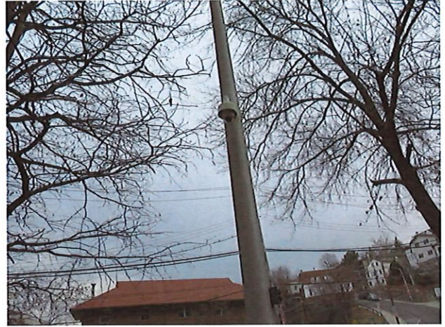
6. Exterior Security Camera
