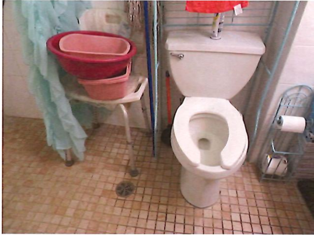
61. UFAS Unit 22 Two Bedroom One Bathroom (occupied): Bathroom No Grab Bars (Critical Repair)
