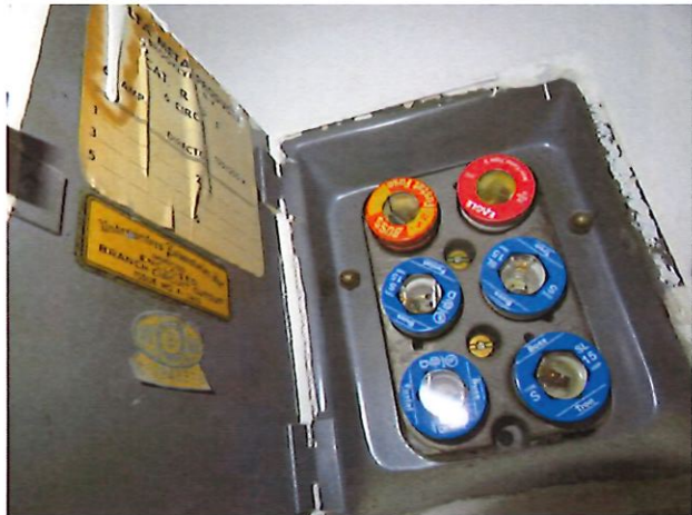
83. Screw-in Fuse (SL/TL) Panel
