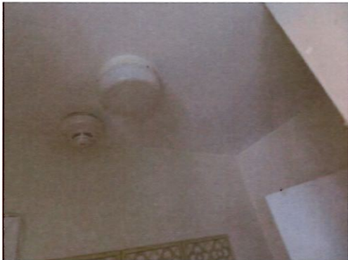
Unit 29 One Bedroom One and a Half Bathroom (occupied): Typical Smoke Alarm
