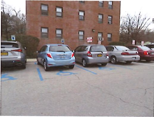
Accessible Parking Near Leasing Office - No access aisles (Critical Repair)
