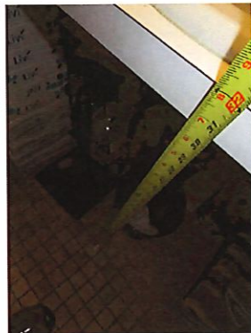
UFAS Unit 22 Two Bedroom One Bathroom (occupied): Bathroom Sink Height
