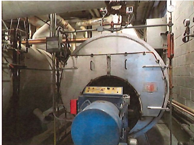
55. AL Eastmond & Sons Boilers
