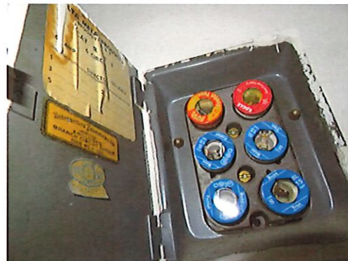
Screw-in Fuse (SL/TL) Panel
