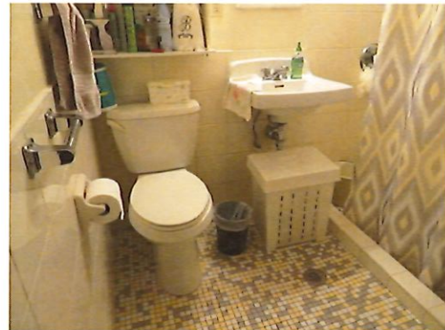
UFAS Unit 103 Two Bedroom One Bathroom (occupied): Bathroom Needs Grab Bars (Critical Repair)
