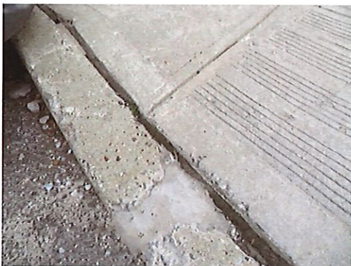
Cracking Ramp Concrete (Critical Repair)
