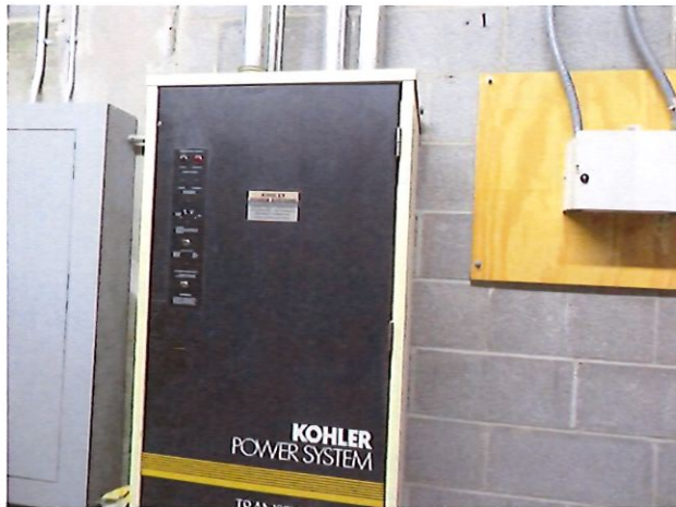
67. Transfer Switch for Generator
