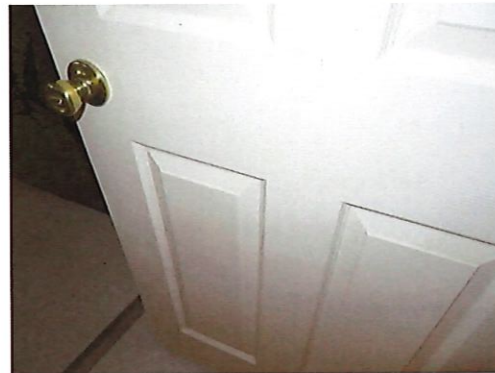
UFAS Unit 103 Two Bedroom One Bathroom (occupied): Bathroom Door Doesn't Have Levered Hardware (Critical Repair)
