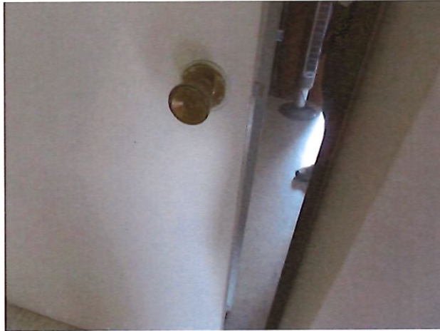
21. UFAS Unit 103 Two Bedroom One Bathroom (occupied): Bedroom Does Not Have Levered Hardware (Critical Repair)
