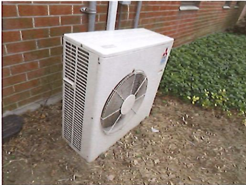
Outdoor Heat Pump Unit
