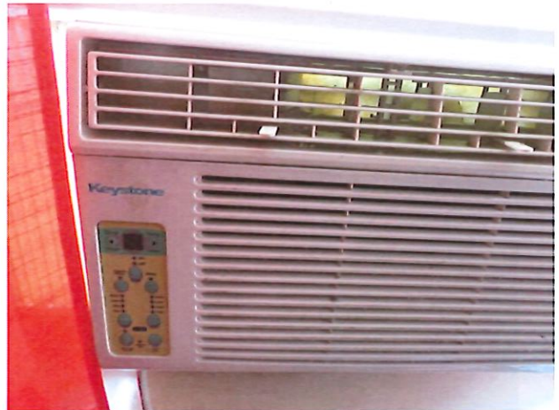
84. Air Conditioning Units
