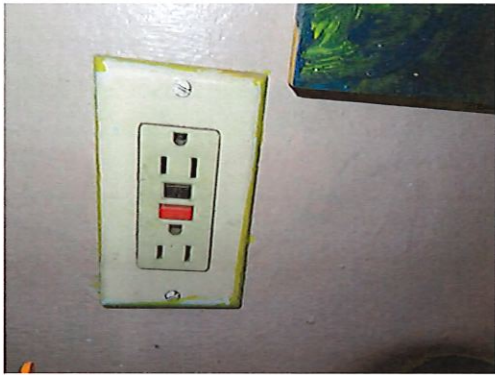
Unit 82 Two Bedroom One Bathroom (occupied): Bathroom GFCI
