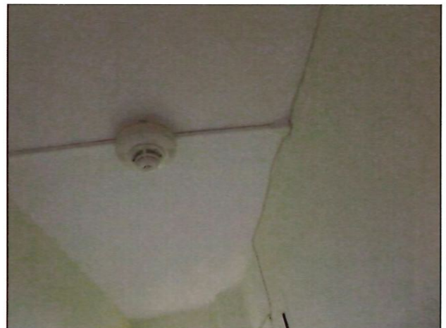
32. Unit 108 One Bedroom One Bathroom (occupied): Typical Smoke Alarm
