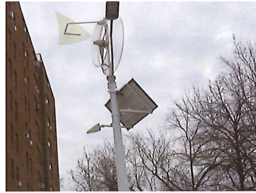
Solar and Wind Generation for Parking Light Fixtures
