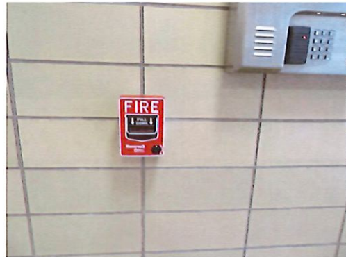
Fire Pull Station
