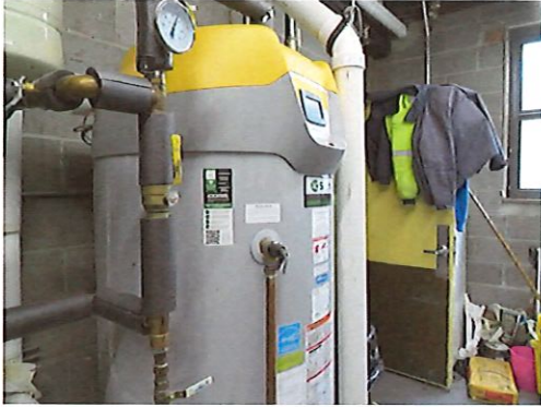
AO Smith Water Heater
