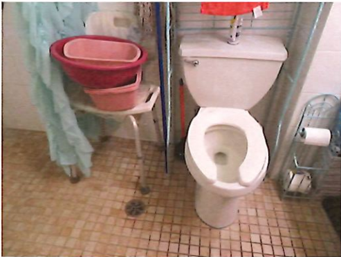
UFAS Unit 22 Two Bedroom One Bathroom (occupied): Bathroom No Grab Bars (Critical Repair)
