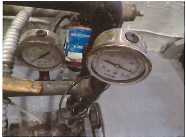
58. Well Pump Pressure Gauge
