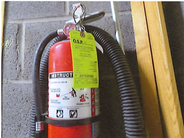
59. Typical Fire Extinguisher
