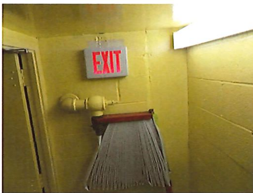
Typical Fire Exit Sign
