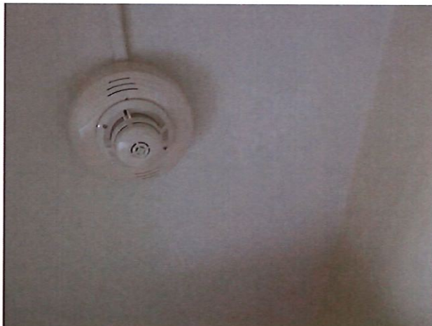
19. UFAS Unit 103 Two Bedroom One Bathroom (occupied): Typical Smoke Alarm
