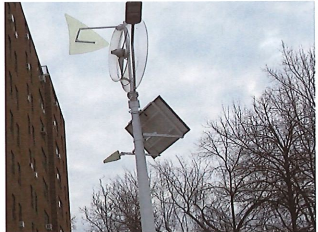
32. Solar and Wind Generation for Parking Light Fixtures
