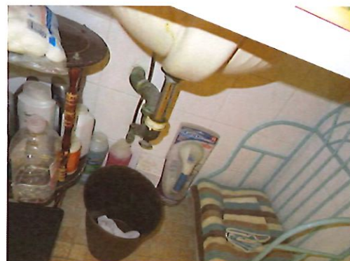
UFAS Unit 22 Two Bedroom One Bathroom (occupied): Bathroom Sink No Scald and Abrasion (Critical Repair)
