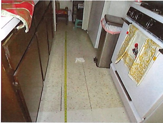
9. UFAS Unit 103 Two Bedroom One Bathroom (occupied): Kitchen Width is less than 40-inches (Critical Repair)
