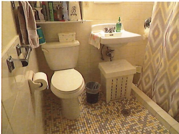
11. UFAS Unit 103 Two Bedroom One Bathroom (occupied): Bathroom Needs Grab Bars (Critical Repair)
