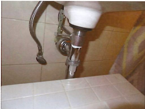
UFAS Unit 103 Two Bedroom One Bathroom (occupied): Bathroom Sink Needs Scald and Abrasion (Critical Repair)
