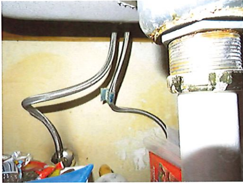
UFAS Unit 103 Two Bedroom One Bathroom (occupied): Sink Under Counter Not Prepped For Wheelchair (Critical Repair)
