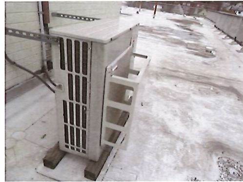
Rooftop Heat Pump Condensing Unit
