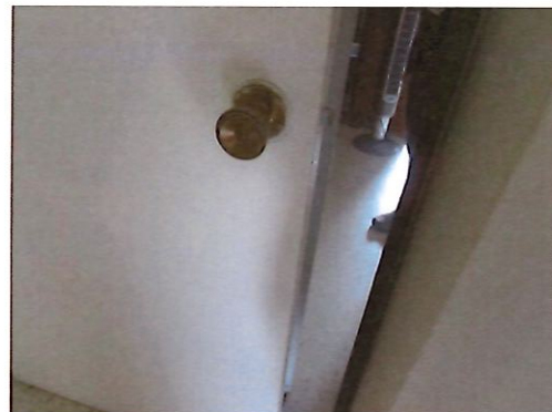
UFAS Unit 103 Two Bedroom One Bathroom (occupied): Bedroom Does Not Have Levered Hardware (Critical Repair)
