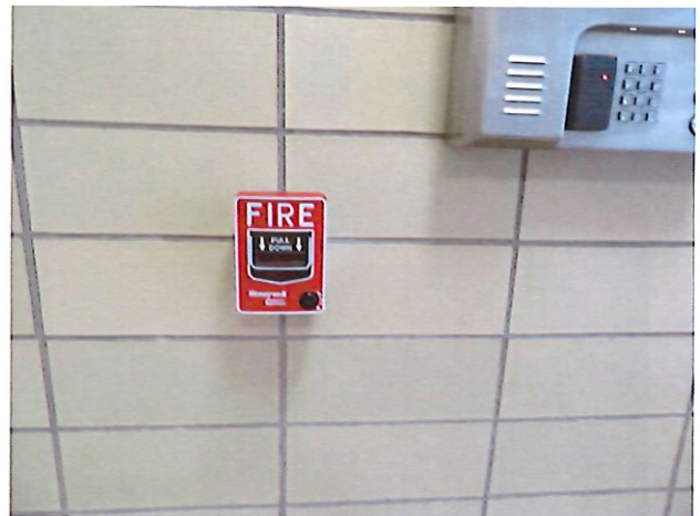
10. Fire Pull Station
