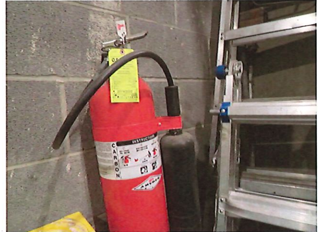
56. Typical Fire Extinguisher
