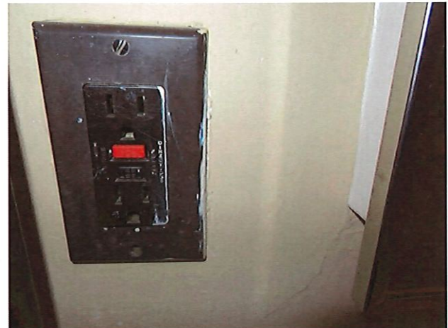
28. Unit 104 Three Bedroom One Bathroom (occupied): GFCI in Bathroom
