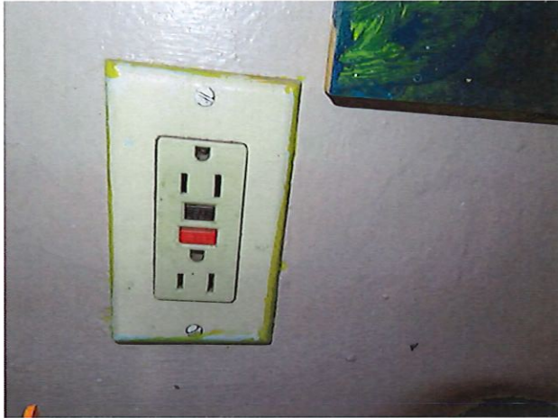
49. Unit 82 Two Bedroom One Bathroom (occupied): Bathroom GFCI
