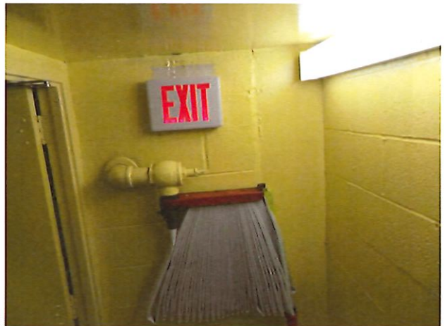
60. Typical Fire Exit Sign
