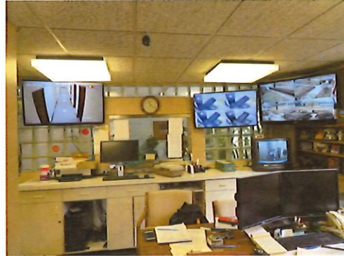
Security Systems Room
