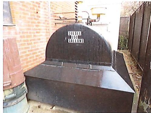
Diesel Tank for Emergency Generator
