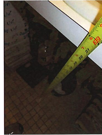
66. UFAS Unit 22 Two Bedroom One Bathroom (occupied): Bathroom Sink Height
