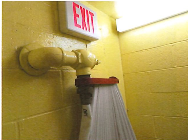
51. Typical Indoor Fire Hose
