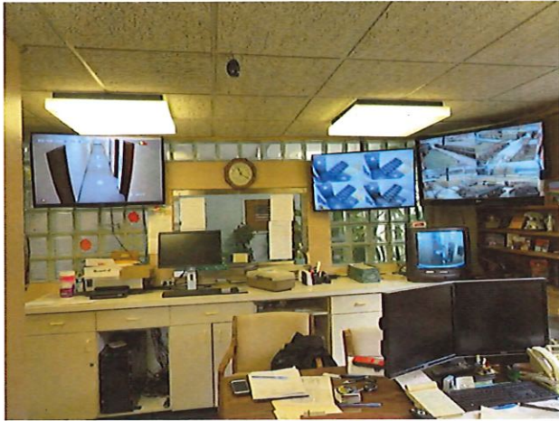
45. Security Systems Room
