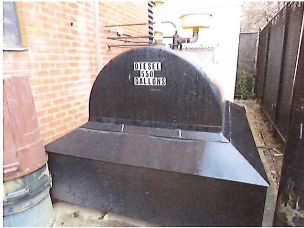
81. Diesel Tank for Emergency Generator
