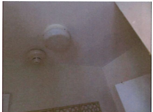
80. Unit 29 One Bedroom One and a Half Bathroom (occupied): Typical Smoke Alarm
