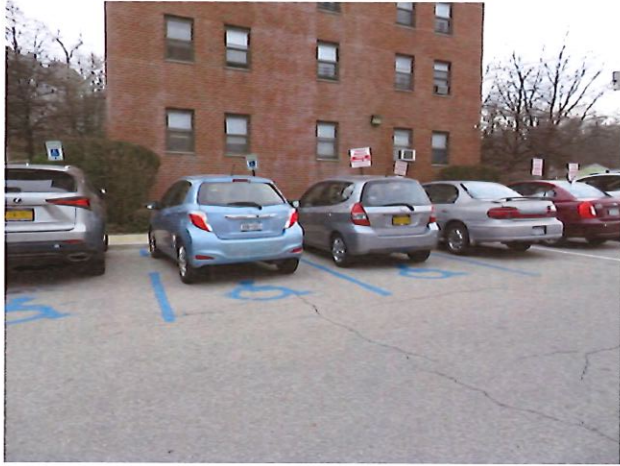
1. Accessible Parking Near Leasing Office - No access aisles (Critical Repair)
