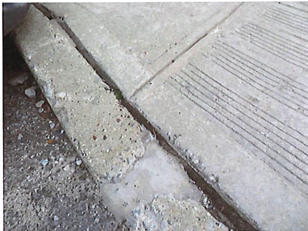
31. Wheelchair Access Way Needs to be Repaired (Critical Repair)
