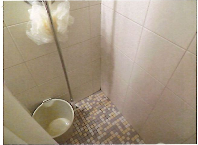
14. UFAS Unit 103 Two Bedroom One Bathroom (occupied): Shower Hose Broken (Critical Repair)
