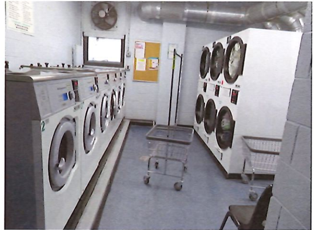
18. Laundry Room Washers and Dryers
