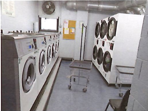
Laundry Room Washers and Dryers
