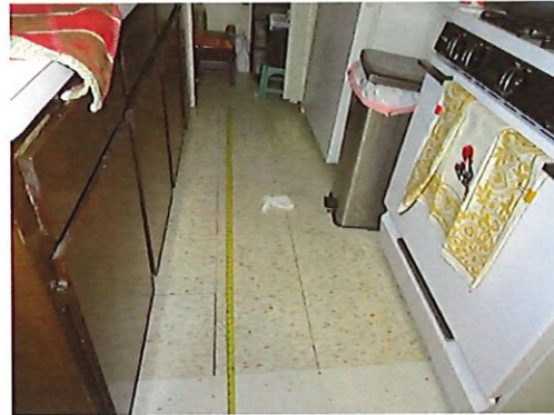
UFAS Unit 103 Two Bedroom One Bathroom (occupied): Kitchen Width is less than 40-inches (Critical Repair)
