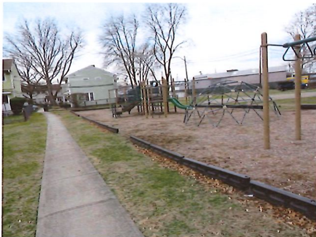
43. Playground Needs Correct Path of Travel to Swings and Slides (Critical Repair)
