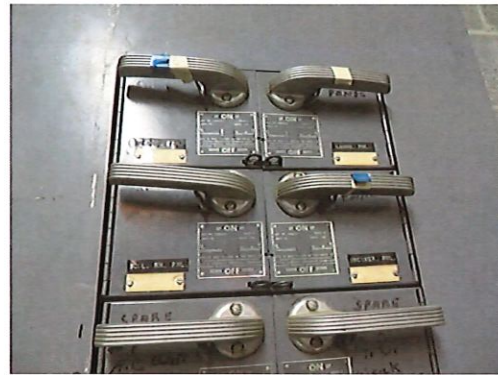
Main Switch Board In Electrical Room
