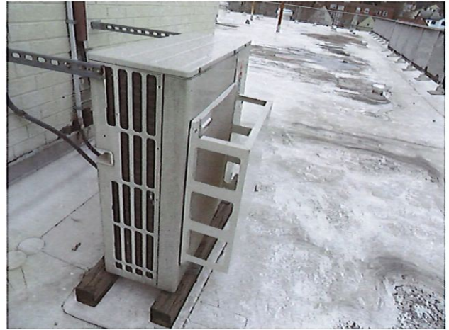
78. Rooftop Heat Pump Condensing Unit
