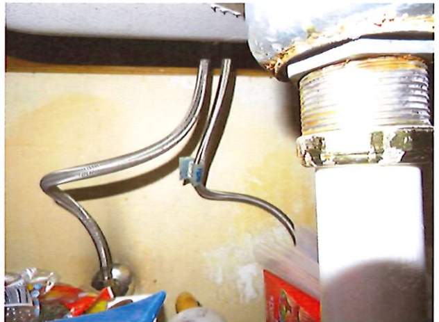
8. UFAS Unit 103 Two Bedroom One Bathroom (occupied): Sink Under Counter Not Prepped For Wheelchair (Critical Repair)
