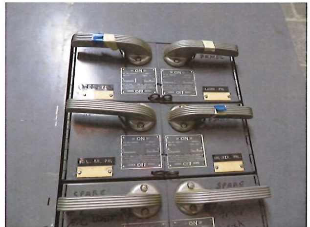
68. Main Switch Board In Electrical Room
