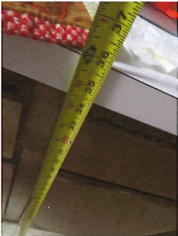
7. UFAS Unit 103 Two Bedroom One Bathroom (occupied): Kitchen Sink Height
