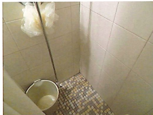
UFAS Unit 103 Two Bedroom One Bathroom (occupied): Shower Hose Broken (Critical Repair)
