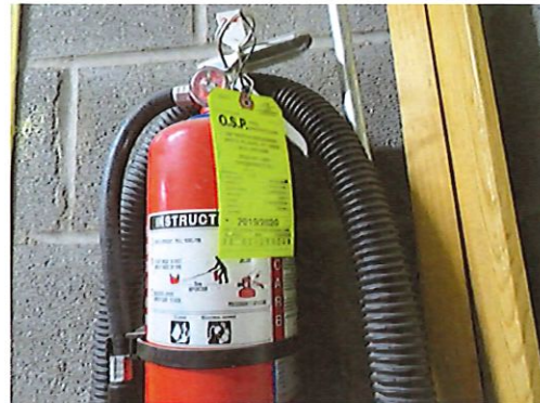
Typical Fire Extinguisher
