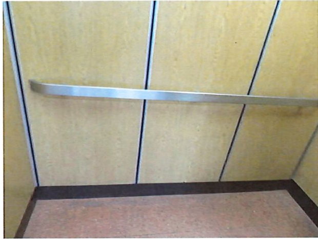
13. Elevator Cab Interior
